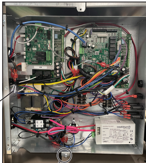
Figure 13B: Wire access (control box closed)
